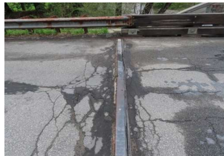
3: Typical gouges in joint (south joint shown). Also, note the pavement breaking up along the joint and the minor approach settlement.
