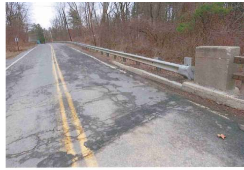
Photo 3: East approach with extensive cracking and areas of settlement.
