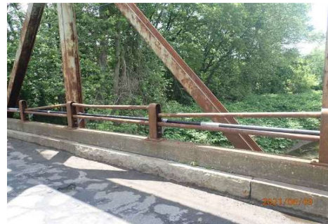
14: South Railing, 10th and 12th panel from West Abutment upper rail disconnected
