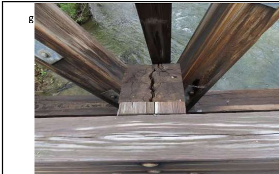
4: Typical splitting in the railing posts and blockouts.
