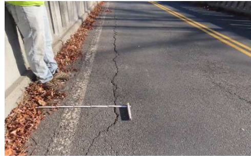
Photo 3: Longitudinal reflective cracking along the north curb, consistent with the misalignment between beams 1 & 2. Also, note the debris along the curbs.
