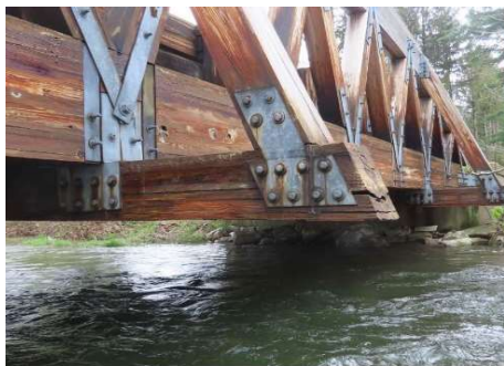
8: Typical splitting and delaminations in the ends of the sway bracing.
