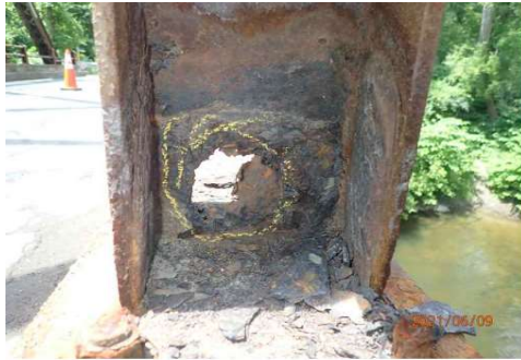
12: North Railing, 11th post from East Abutment with perforation in low web
