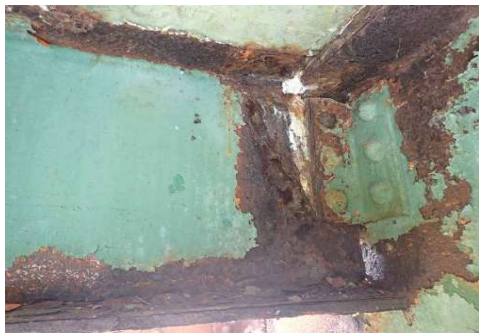
21: Stringer S5 at Floorbeam FB3, north face with rust and section loss
