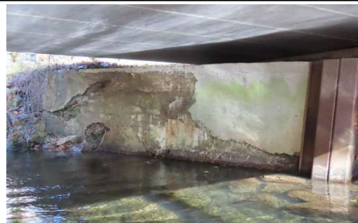
Photo 6: Old abutment wall at the east side showing extensive cracking, efflorescence and scaling.
