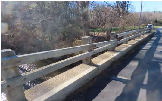
Photo 5: South railing with detached rails.
