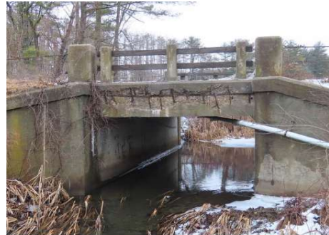
: Spalling throughout the west fascia (rail base and frame roof).
