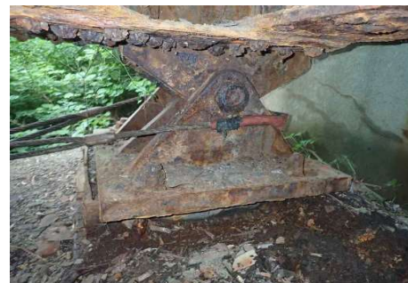
42: Southwest Bearing with debris, rust, and anchor bolt nut section loss as well as overexpansion with bent anchor rods
