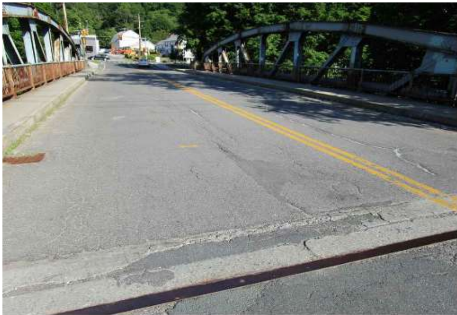
3: Typical Wearing Surface, Heavy Alligator and Longitudinal Cracking and Patches, Looking East
