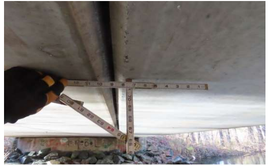
Photo 4: Vertical misalignment between beams 1 & 2.
