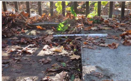
Photo 4: East approach sidewalk showing settlement adjacent to the bridge.
